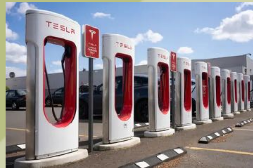
Public DC Fast Charger L3 - Main Battery DC Voltage
